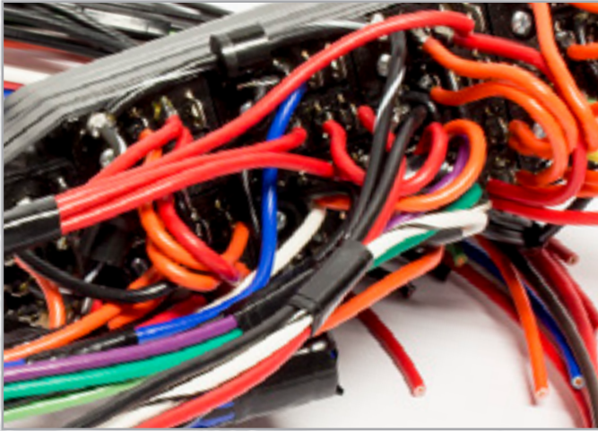
Before: Bundled random relays and a multitude of tangled wires.
